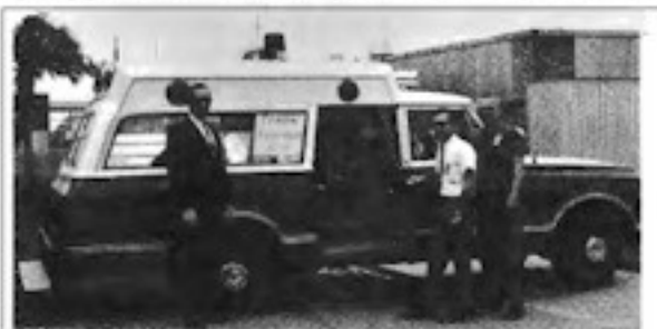
John McQueen, Marshall DuBois, Andy Foppe installed EKG telemetry system in South Trail ambulance.
