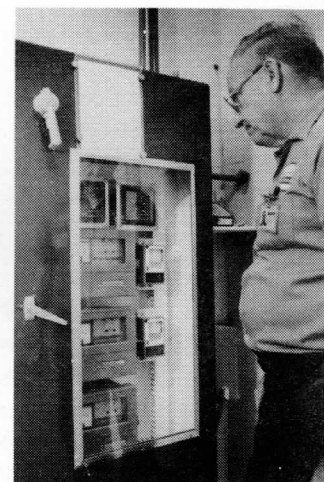
Harry Yates with control panel for industrial pre-treatment system.
